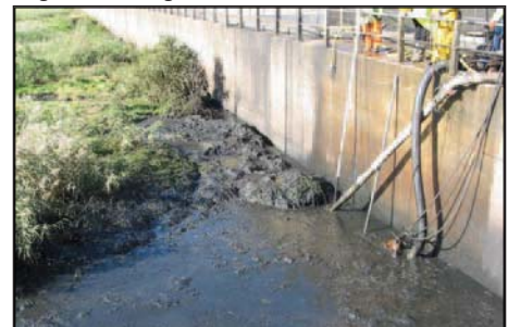
Settlement Tank Clearing - Chopper Pump
